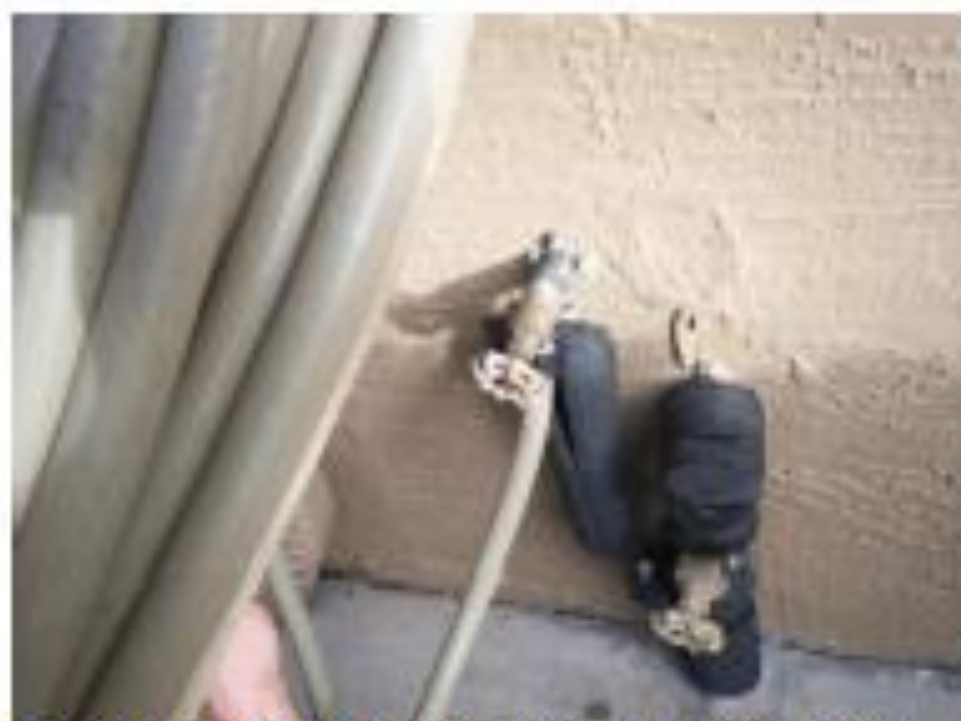
Photo 1- The main water shut off at the right exterior of the garage.
