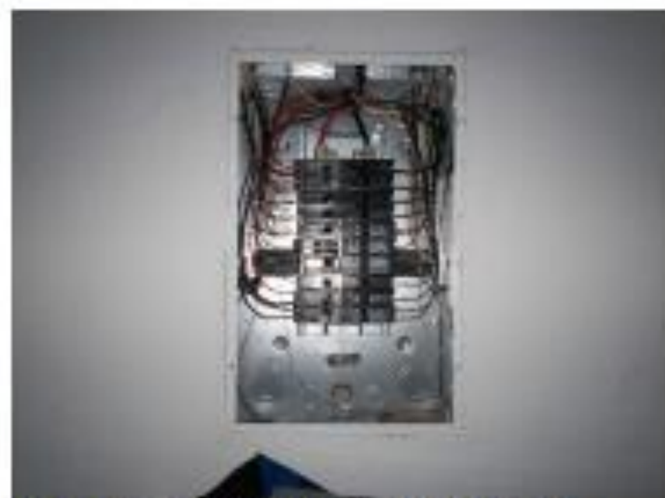
Photo 3- The Cutler Hammer Brand distribution panel in the garage.
