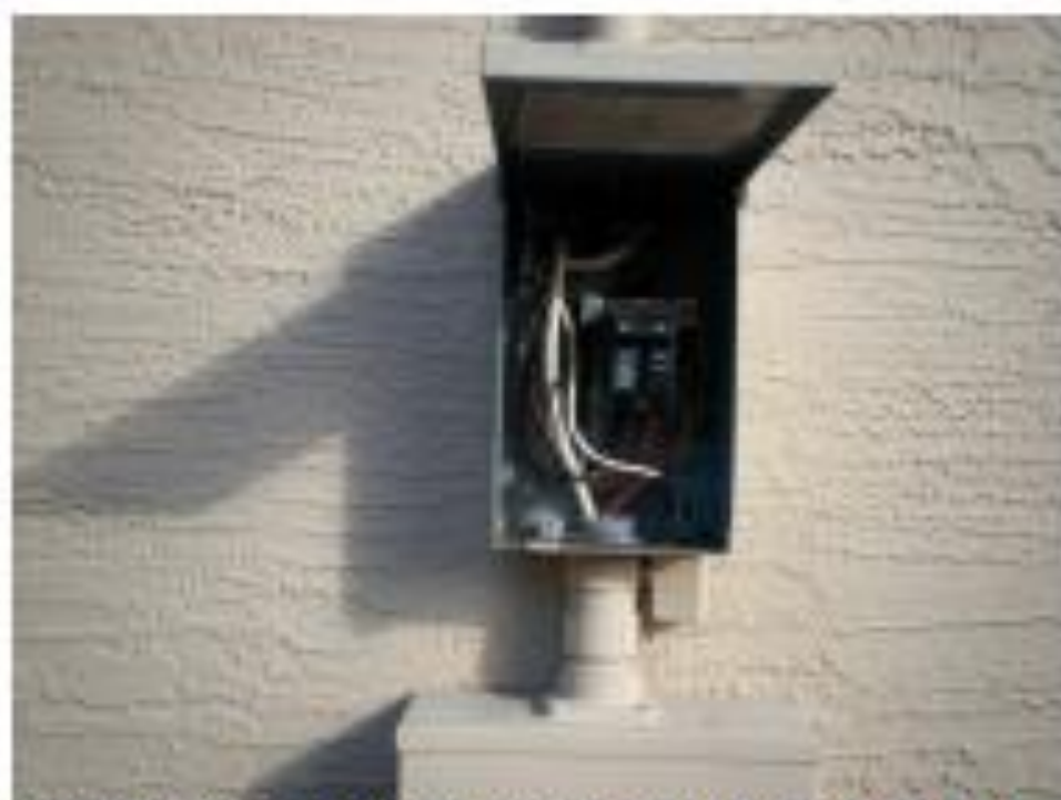
Photo 2- The Cutler Hammer Brand 125 amp main disconnect panel at the right exterior of the garage.
