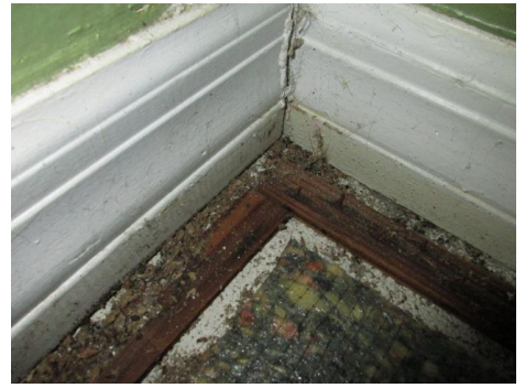
Moisture stains on tack strips
