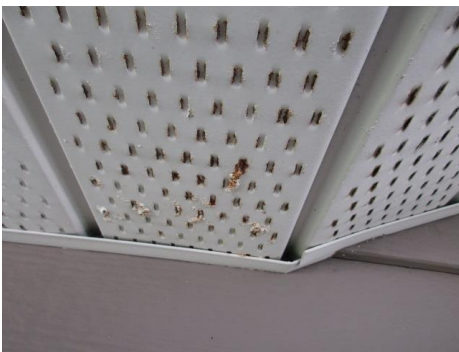
Corrosion under cut drip edge
