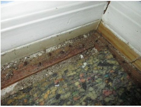
Moisture stains on tack strips
