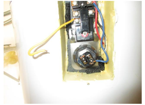
Damaged wire, prior to my repair
