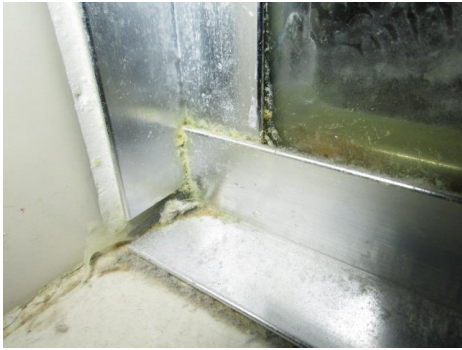
Evidence of moisture escaping shower at window
