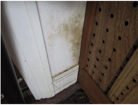
Moisture stains, garage near water heater
