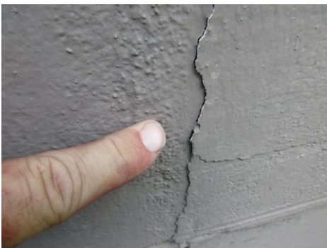
Crack at frame repair
