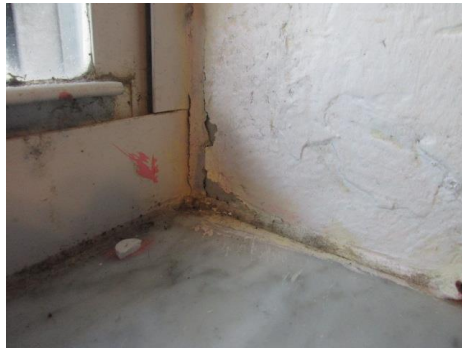
Moisture evidence on window
